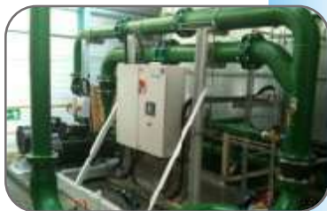
Air Conditioning Plant
